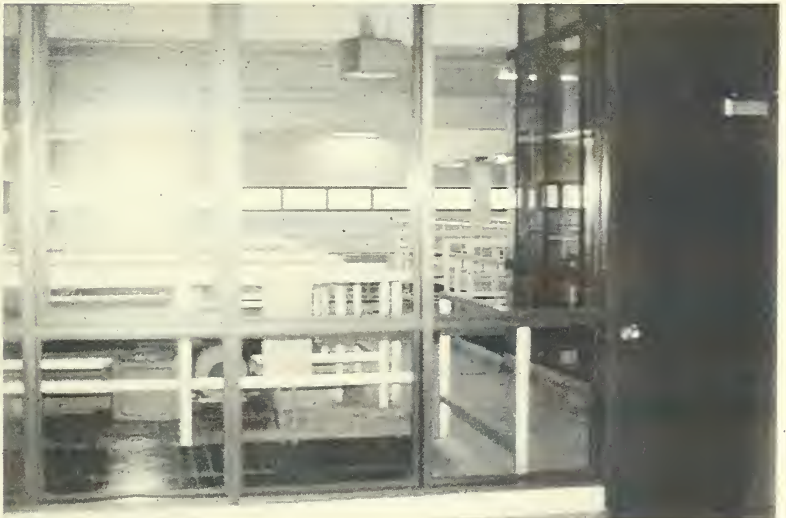
6. VIEW OF FLOCCULATION TANKS FROM CONTROL ROOM
